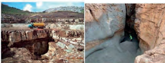
Figure 5: Major cavities encountered in the Balaa dam basin and attempt to seal them with cement (ZAATITI, 2017)
