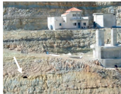
Figure 3: Open karst feature on the right embankment of Chabrouh Dam (visible on the lower left corner of the picture).
