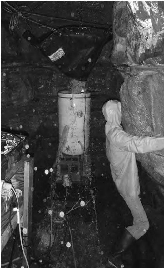
Figure 3. Discharge barrel and data logger setup at WF1 during storm event.
