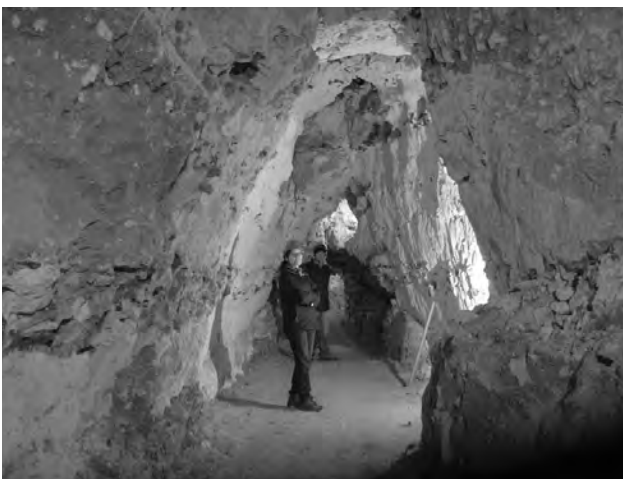
Figure 7. Flooding reservoir resulting of coalescence of several equilibrium chimneys developed on the structure, obliquely to the axis of the drain, between pt. 26 and pt. 24 (photo by J. Rodet).
