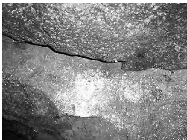
Figure 2. White leucite crystals clearly visible in a slab of rock in Sugano 2 tunnel.
