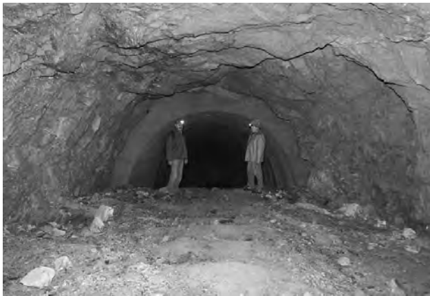
Figure 3. The unfinished crown of the tunnel. The section in the background has already been lined with concrete.
