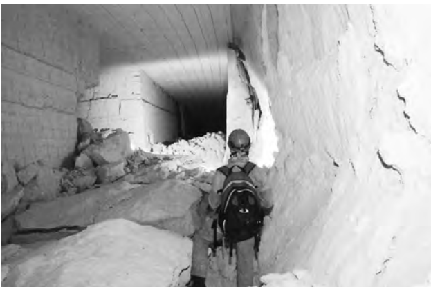
Figure 4. Lateral failures from the wall in a calcarenite quarry. Note the development of linear sliding surfaces.
