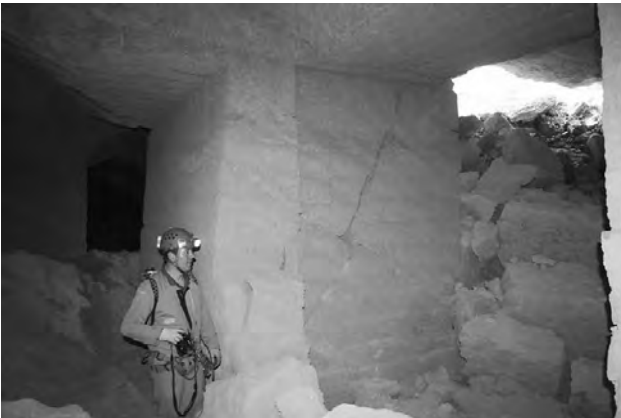
Figure 7. Cracks crossing a pillar, along primary (clino-stratification, dipping to the right in the picture) and secondary (open cracks) discontinuities.
