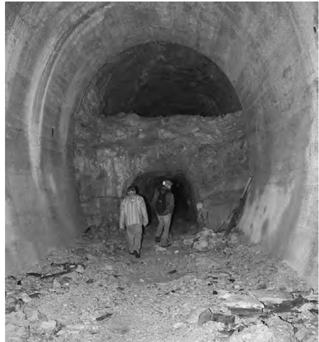
Figure 4. View of the pioneer tunnel and crown section and a section of nearly finished tunnel.
