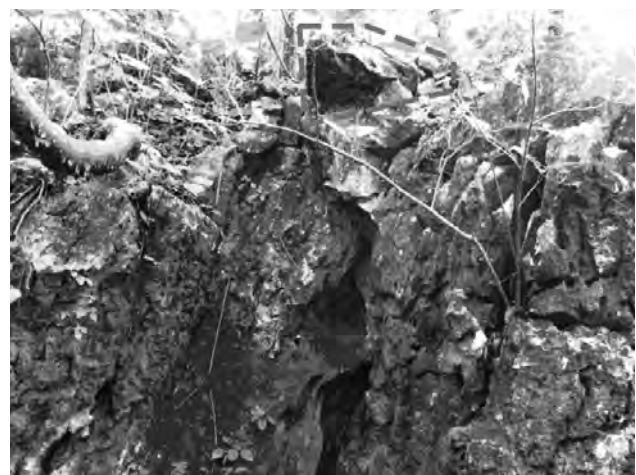
Figure 4. Zone of instability in the surface near the cave entrance: unstable rock that may fall inside the cave (Photo: G. Quesada).
