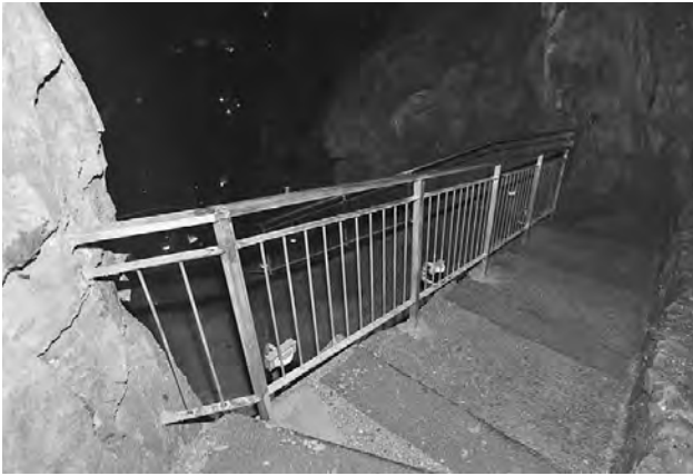
Figure 3. Railings, banisters and parapets of stairs with vertical posts and emergency lights. Photo by A. Fabbriatore.
