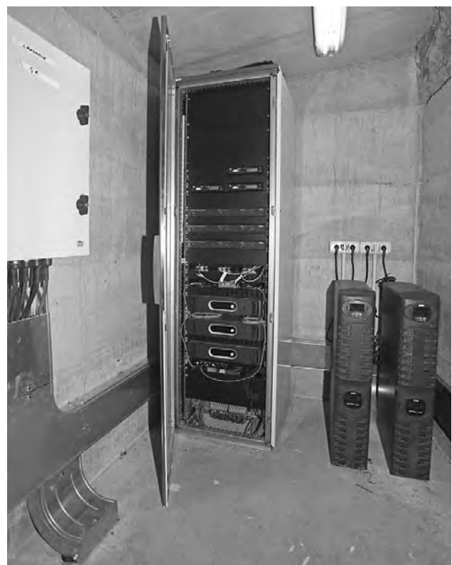
Figure 6. Technical room. Photo by A. Fabbricatore.
