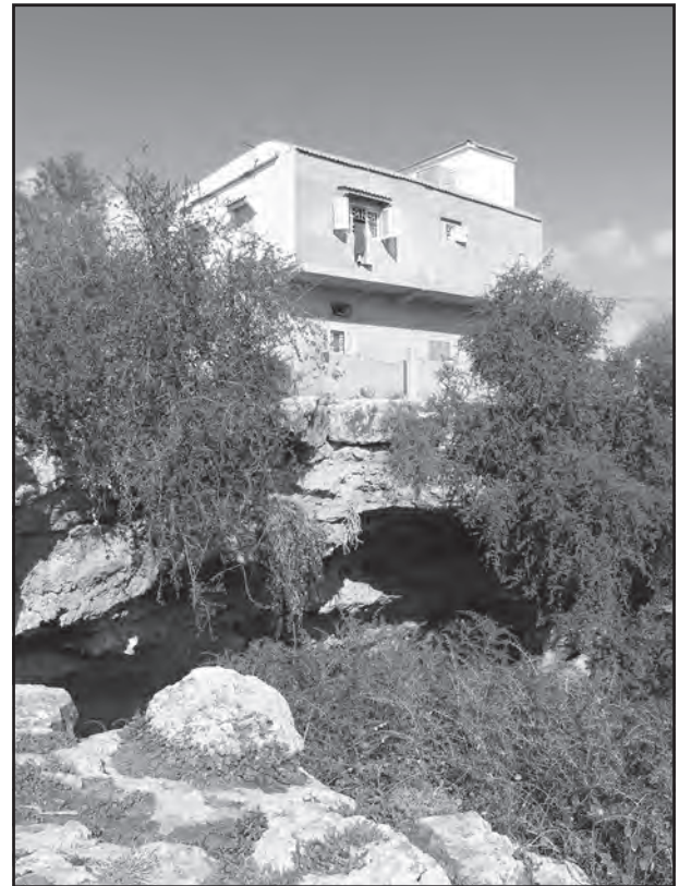
Figure 3: Building over the thin ceiling of Jabbah cave in the karst plain of Benghazi (photo by R. Ruggieri).
