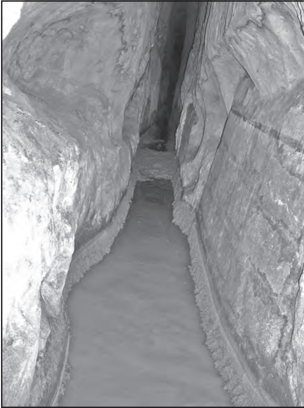
Figure 3: The main tunnel in the Triglio aqueduct (Taranto province, Apulia), one of the longest inventoried aqueducts in southern Italy, with a length of approximately 18 km.
