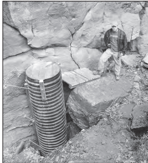
Figure 4: A culvert pipe was placed over the newly opened fissure to prevent large flood debris from sealing the entrance.
