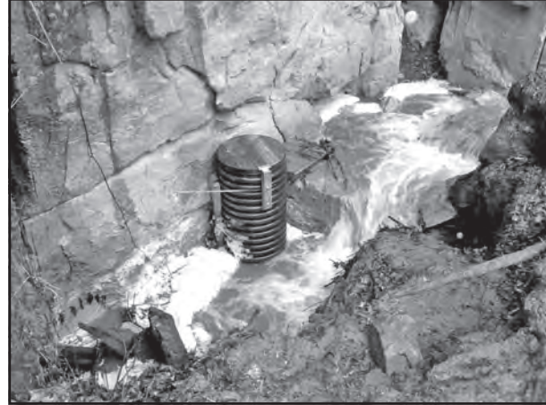
Figure 8. Heavy rains begin flooding that will soon cover the entrance pipe to a depth of 2 meters.
