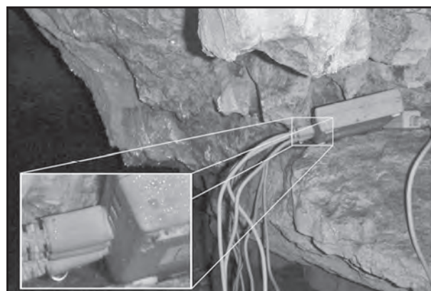
Figure 5: Condensation droplets in CSB Passage. Moisture on the logger (inset) demonstrates that the droplets formed during the study period.
