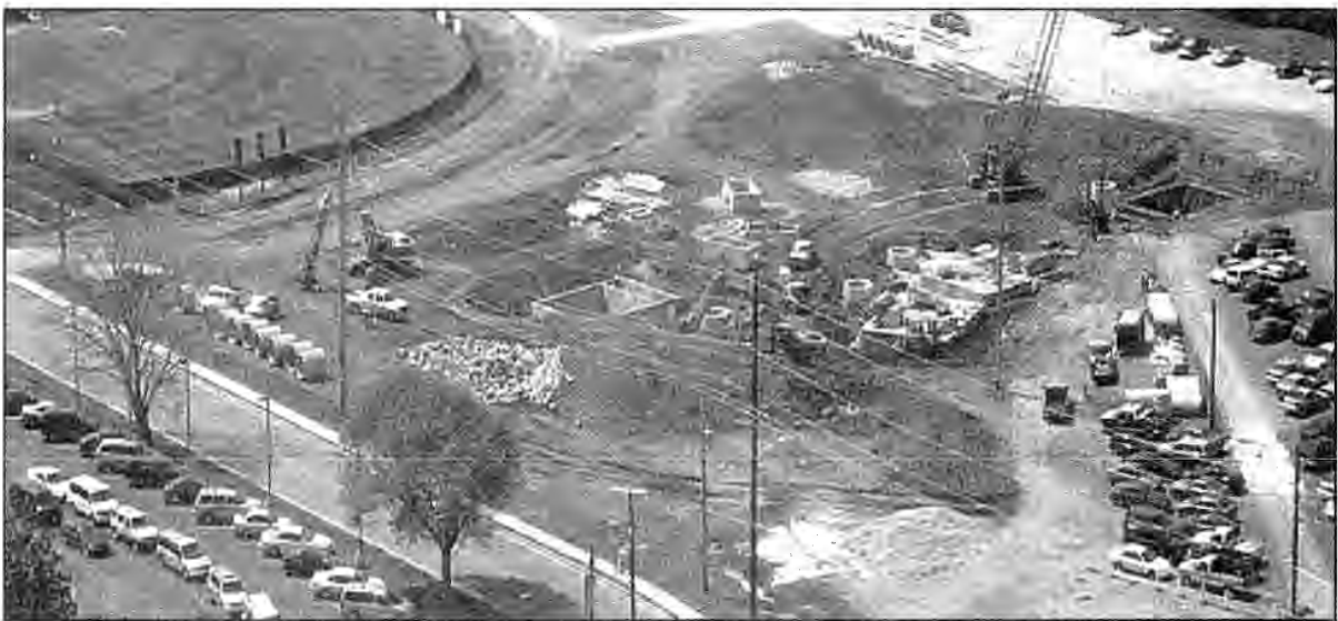
Figure 2. Aerial view of 4 Vortechs units being installed to treat storm water runoff before it is discharge into the Lost River through four 1.22 m (4 ft) diameter wells. Photography courtesy of Vortechtechnics, Inc.
