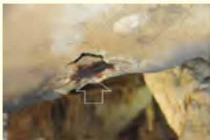
Photo of an area below a trail where the iron has rusted, resulting in damage to the concrete.
