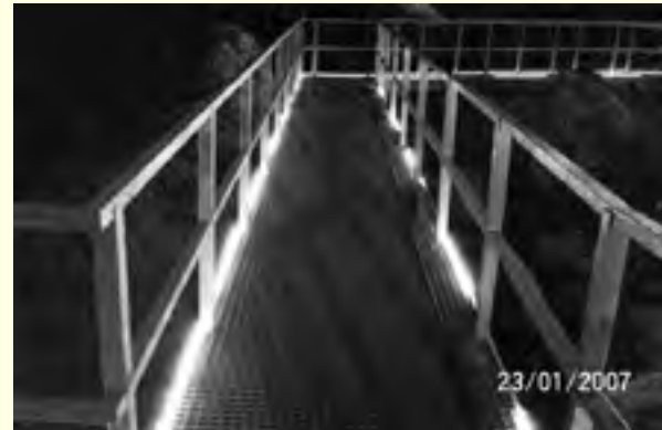
Figure 4. The emergency lights placed along the edge of the pathway in the Grutas de Bustamante, Mexico (Photo Cigna).
